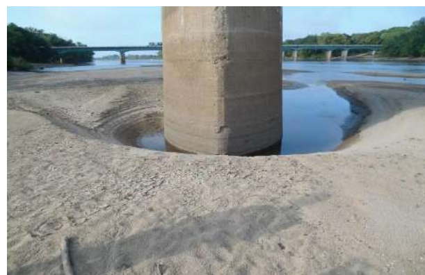
Figure 1: Scour hole around bridge pier [4]
