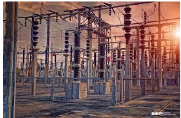
Figure 4: Substation where chances of fault are so much
