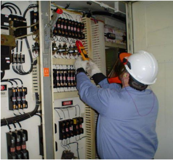
Figure 2: Electrical Equipment Maintenance a Power Panel
