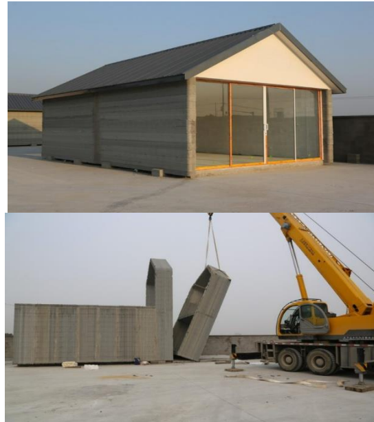
Figure 5: Houses produced with a 3D printer designed by WinSun as a prototype [41]
