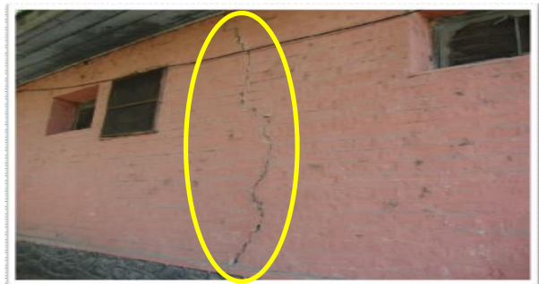
Figure 2: G3 Crack in wall
