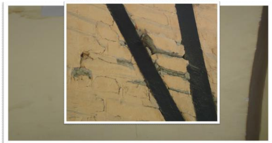
Figure 3: Distress fine crack
