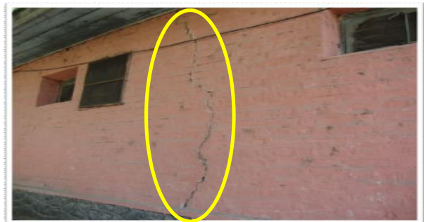
Figure 2: G3 Crack in wall
