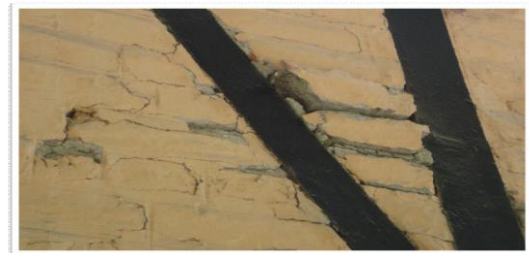
Figure 5: Damage to infill walls
