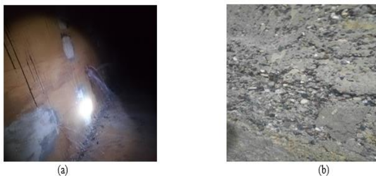
Figure 5: (a) Leakage Between The Pores of The Water Tank, (b) The Surface of The Concrete In The Water Tank
