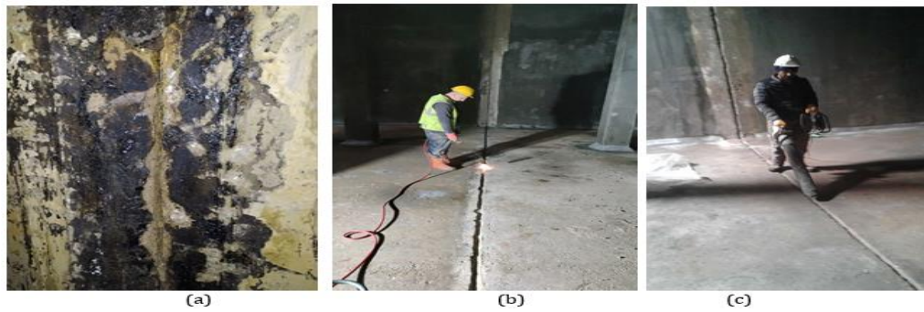
Figure 7: (a) Initial Condition Dilatation Joint, (b) Cleaning The Dilatation Joint With Blowtorch, (c) Cleaning The Dilatation Joint With Air Compressor
