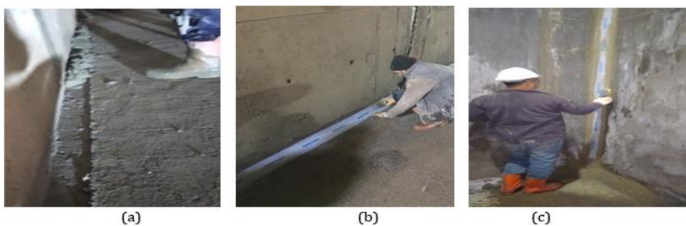
Figure 6: (a) Wall and Base Junction of The Water Tank, (b) Horizontal Chamfer Application, (c) Vertical Chamfer Application
